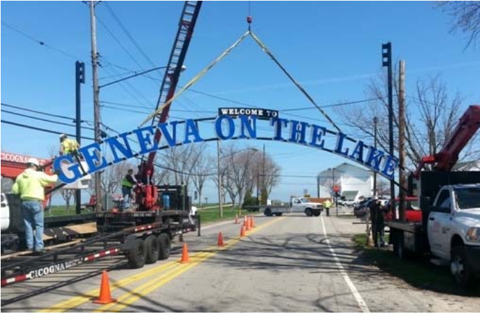
Workers from Cicogna Sign Hoist “Welcome” Sign Over State Route 534 Near the State Park Lodge
